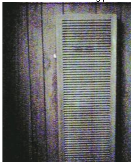
the modern heating plant
